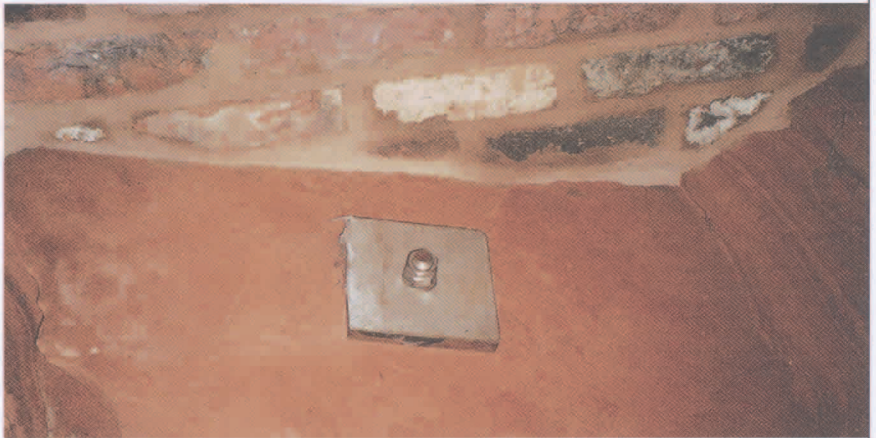
Roof bolt support to ballroom ceiling.
