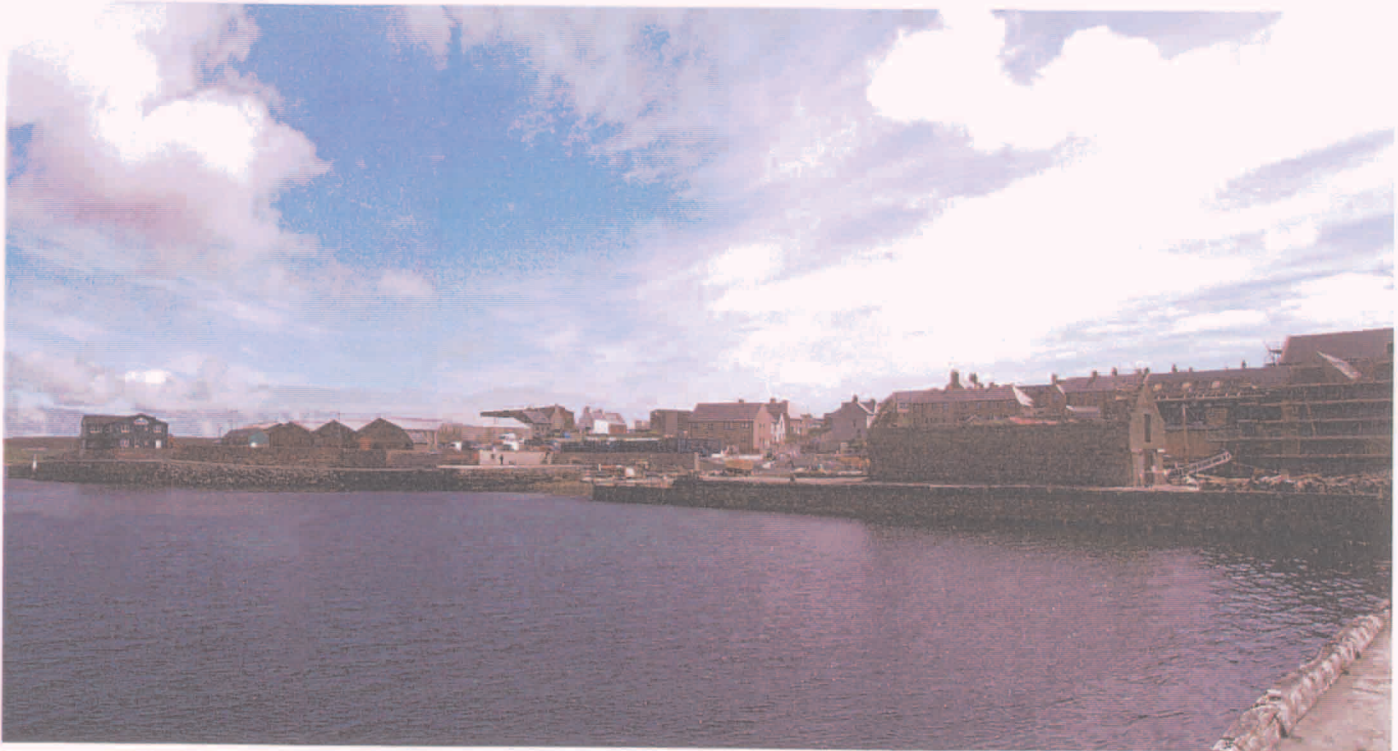
Panorama of Hay's Dock with the Heritage Centre under construction in the background (right), the restoration of the old sail house on the quay (centre right) and Cintec stabilisation work (end of the quay left of sail house)
