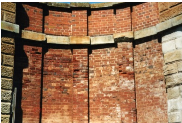
Damage to wingwall — note coloured cement render from 1930s and salt deposition caused by it.
