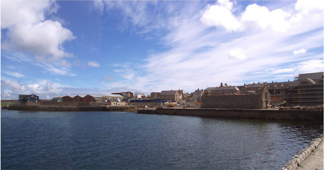
Panorama of Hay's Dock with the Heritage Centre under construction in the background (right), the restoration of the old sail house on the quay (centre right) and Cintec stabilisation work (end of the quay left of sail house)
