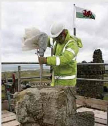
Diamond drilling to install anchors to secure stonework to high level chimney stack
